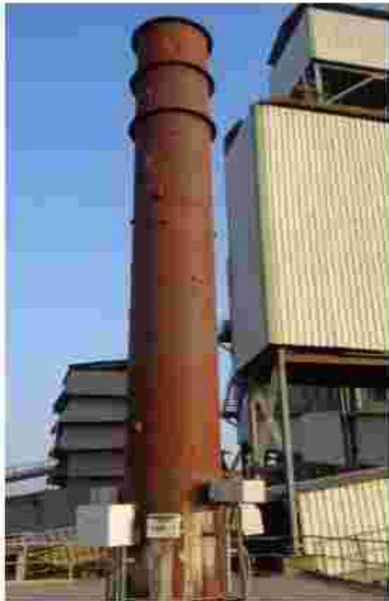
CEMS in the stack of Bag House of Cement Mill-3, Imtal
