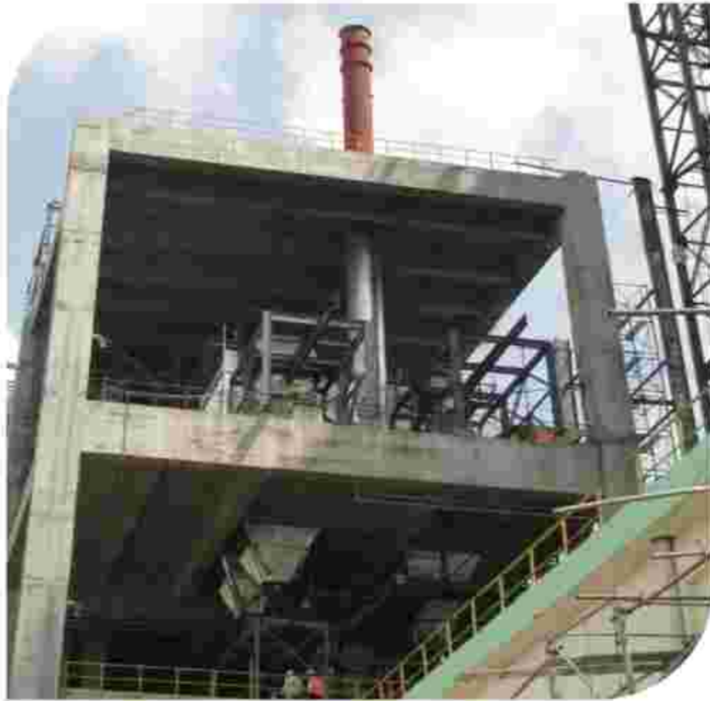
Bag House of Cement Mill-3 along with stack
