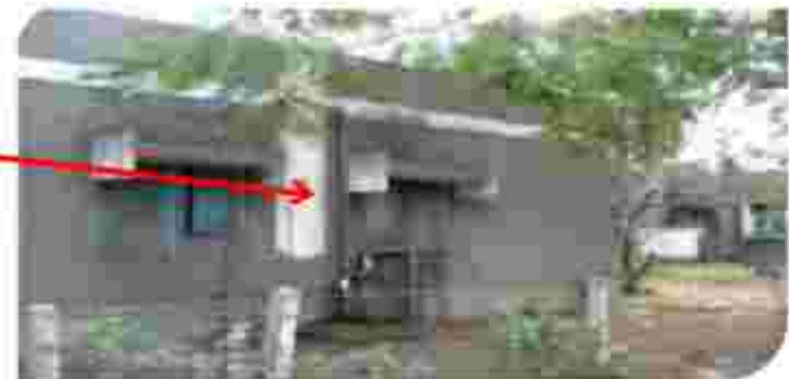
RWH Filter at 11 th Block Quarter – Colony in Imlai
