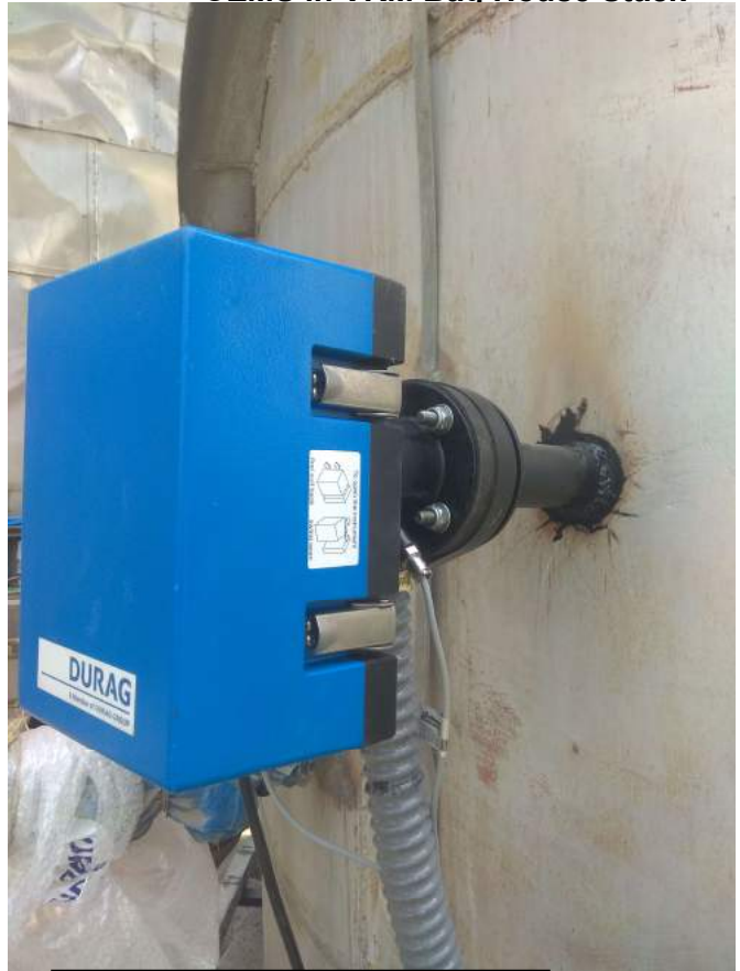
CEMS in VRM Bag House Stack
