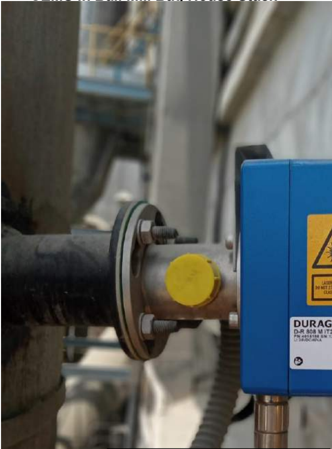
CEMS in Ball Mill Bag House Stack
