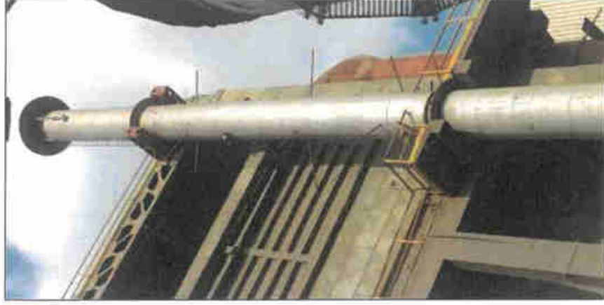
Bag House of Ball Mill along with Tall Stack
