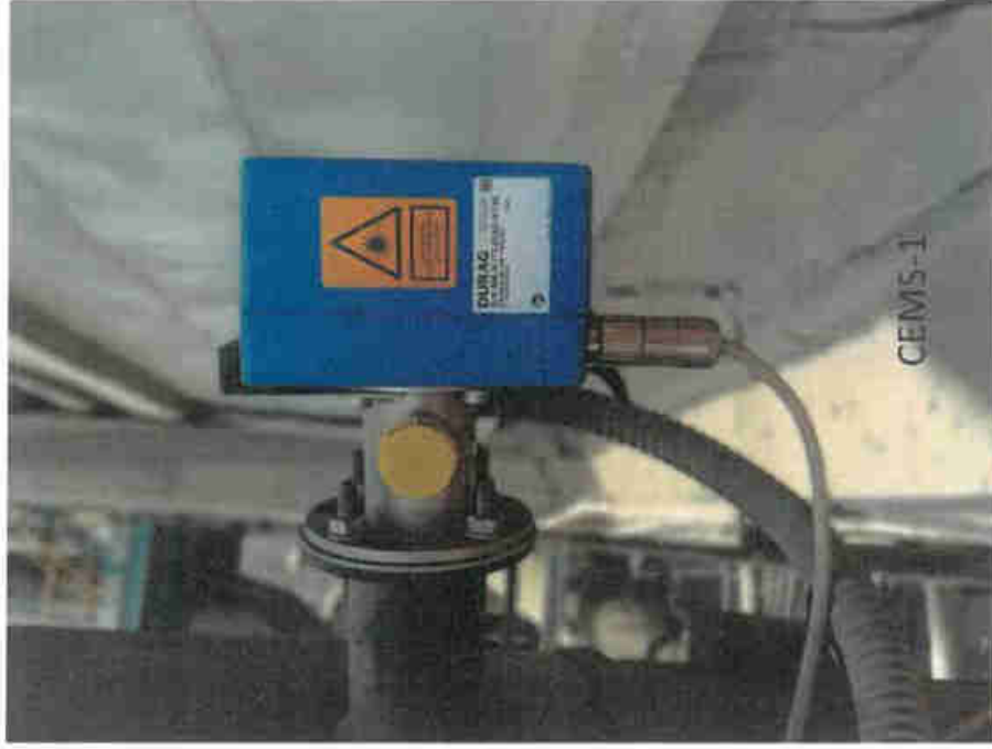
Annex.-4(Online CEMS in both Stacks)
